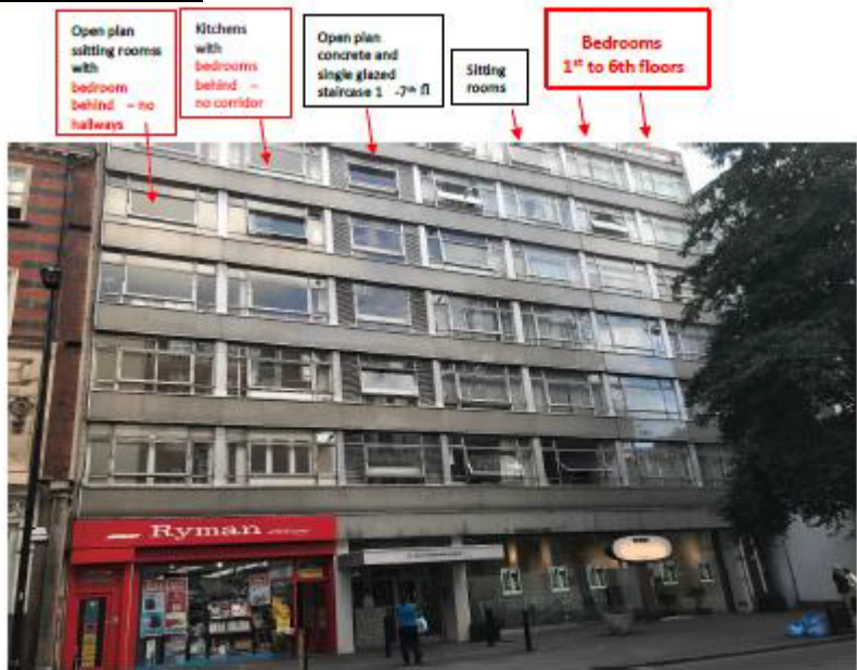
Front elevation 89 GPs W1W 7LX single glazed 1950's concrete construction over 7 floors showing positions of bedrooms and living spaces in flats on 1 st - 6 th Floors - 12 flats single aspect and all single glazed.
